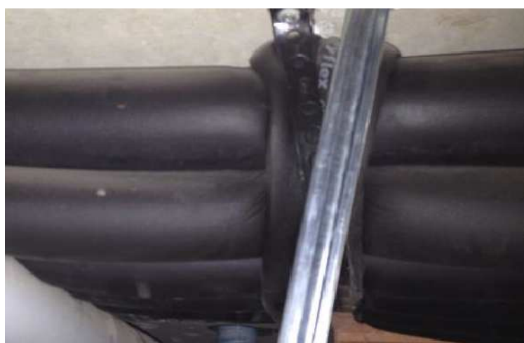
Example of pipe support reducing thickness and crowded pipes thickness
