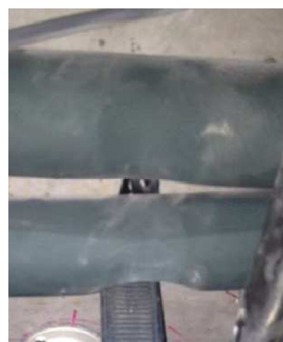
Pipe support reducing insulation
