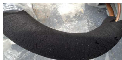
Prolonged exposure to the sun and environment causes cracks
