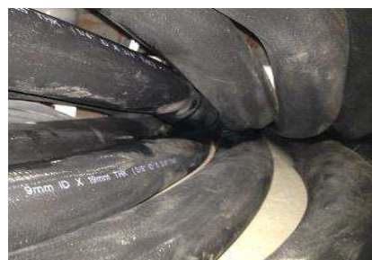
Example of crowded pipes
